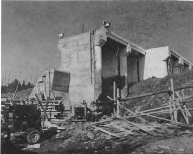
PLATE I — Upstream view showing details of spillway, such as the profile, vertical keyways, steel frame and elevation of pillars.
