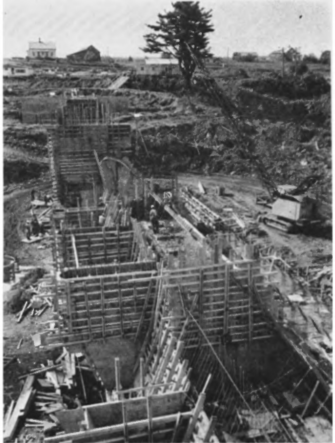
PLATE III — General view, toward the west, showing the erection of coffer, according to the method of successive lifts.
