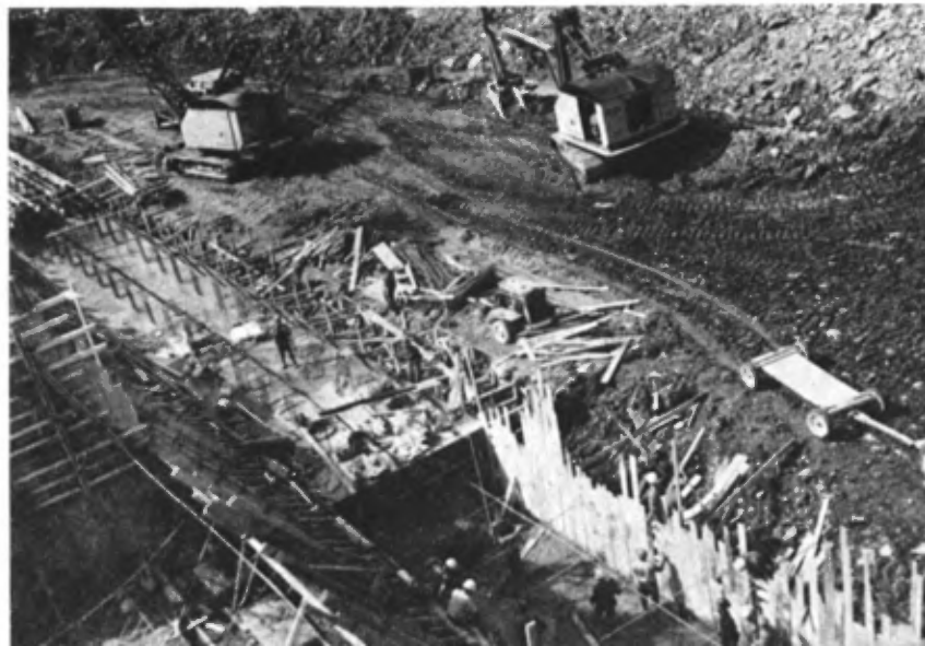
PLATE IV — Detail of the downstream, apron slabs, energy dissipators at three different stages of construction.
