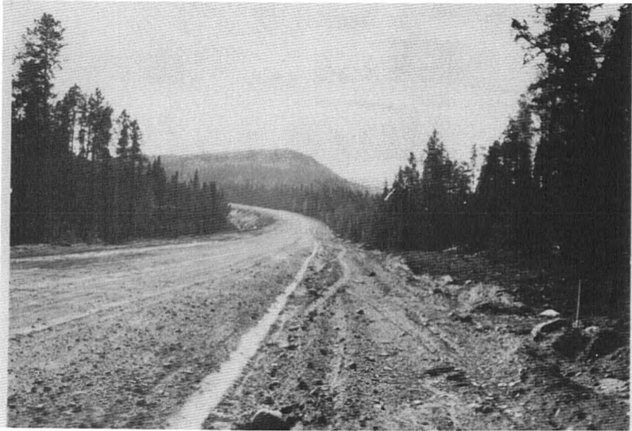
Profile of a typical elongated ridge . The steep slope of the ridge faces west . Highway No. 58, mileage 52 .
