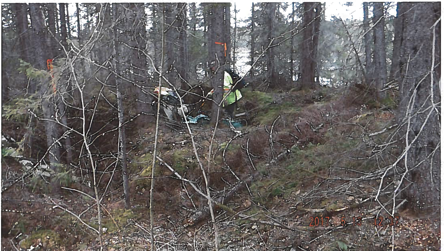
Photograph 2: Hand digging to access bedrock in historic pits located adjacent to Lac Chev.
