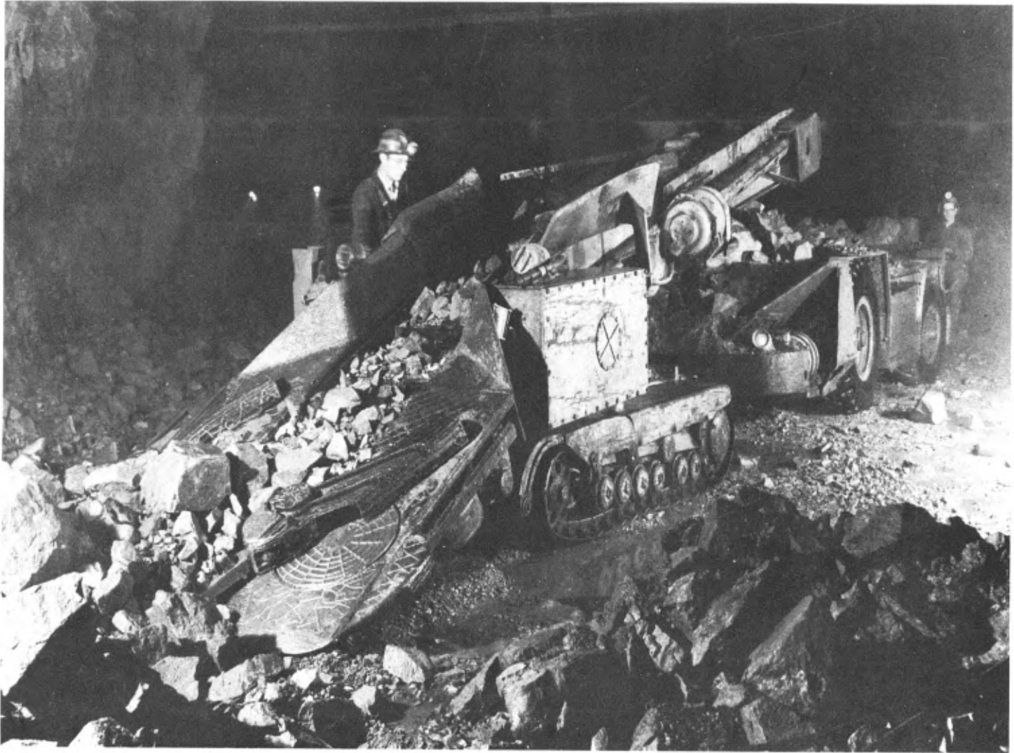
Rock loader and electric shuttle car, at Gaspé Copper Mines Ltd. (Photo: Gaspé Copper Mines Ltd.)
