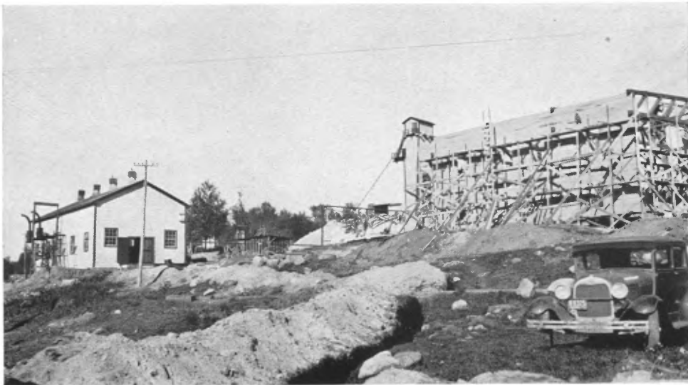
B.—Canada China Clay Company. St-Rémi-d'Amherst, Papineau County. Mill under construction, headframe of the shaft and Power House, 1937.
