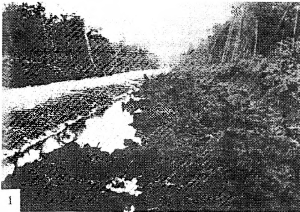
Fig. 1. Heave and displacement from end tipping into peat.
