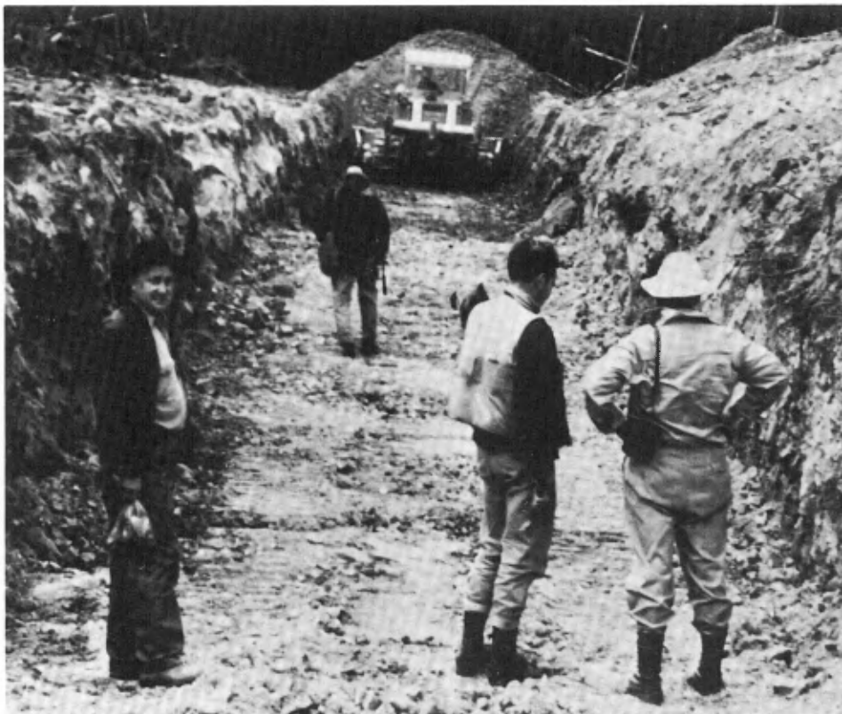
Bulldozer tears open overburden on the Lornex property being explored by Rio Tinto Canadian Exploration, Rio Algom's exploration arm.
