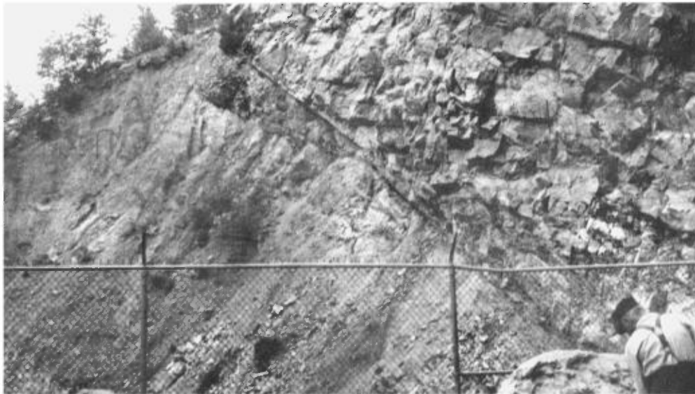
Fig.6 : Fault near the power-house at LaTuque. Taken from same place as above, but looking north.
