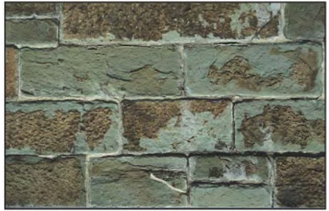
Scaling of bushhammered Sillery sandstone with vertical bedded plane, Fortifications wall.
