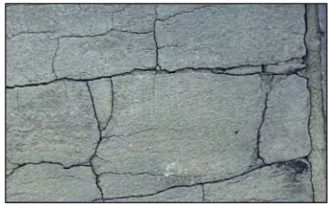
Cracking in Deschambault Formation limestone from Pointe-aux-Trembles, Wolfe-Montcalm Monument.
