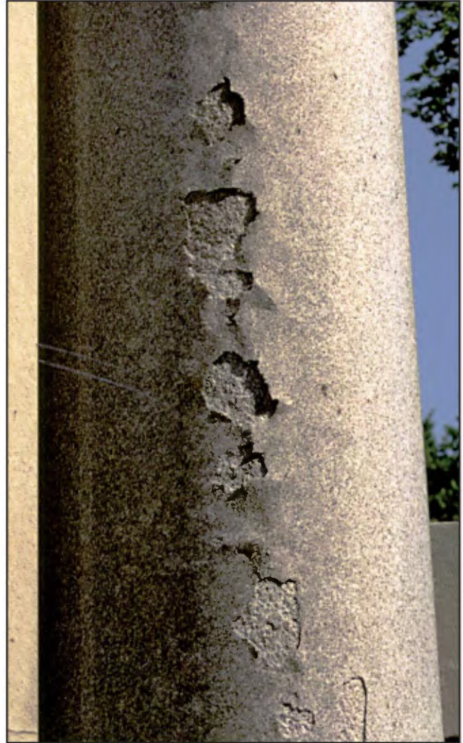
Peeling of a column in Stanstead granite, 20 Pierre-Olivier-Chauveau Street.
