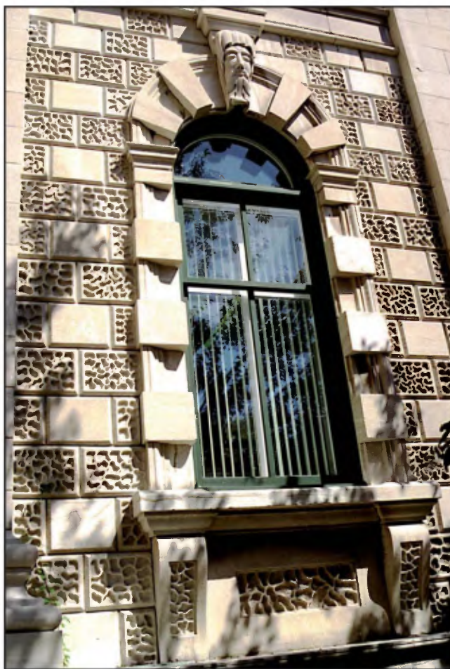
Customs Building: mask, voussoir, jamb, consoles, piers and vermiculated blocks in Saint-Marc-des-Carières limestone.
