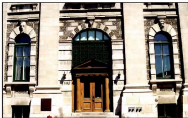
Customs Building: stone facing, vermiculated dressing and mask in Deschambault Formation limestone from Saint-Marc-des-Carières.
