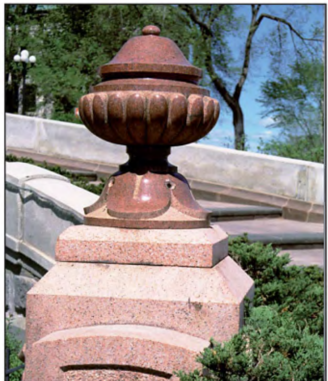
Ball and pedestal in red granite from St. George, New Brunswick. Parapet in Stanstead grey granite, baseboard in “Vieil Or” granite, stair run in “Tadoussac” gneiss and nosing in “Péribonka Black” anorthosite.
