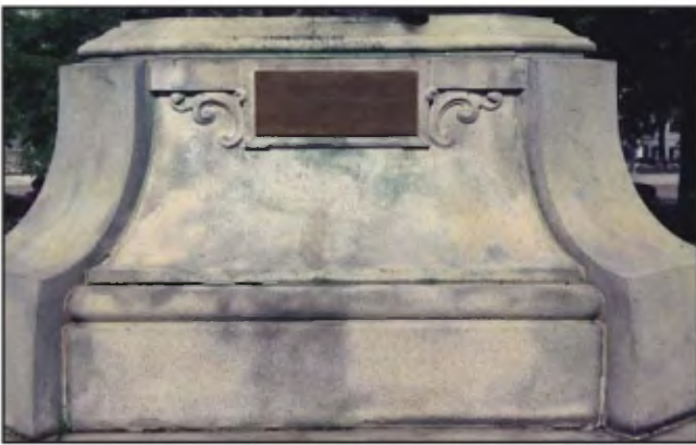
Colored patterns on Stanstead granite caused by adsorption of flowing corrosion products from bronze statues of the Honoré-Mercier Monument.
