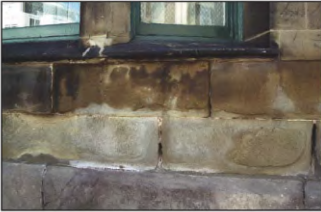
Disintegration and oxidation of the Bouctouche sandstone, N.B., 1 des Grisons Street
