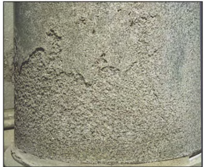
Disintegration at the base of a column in Stanstead granite, 20 Pierre-Olivier-Chauveau Street.
