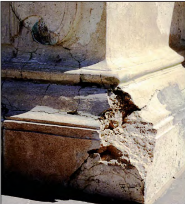
Cracking and disintegration of the Château-Landon limestone from France, Champlain Monument.
